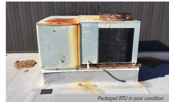
Packaged RTU in poor condition
